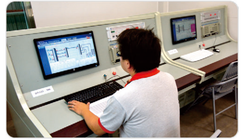
Control room & Graphical HMI
